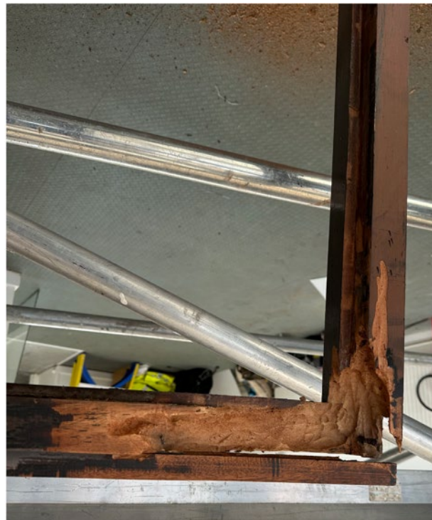
Window removed from frame and rot discovered
