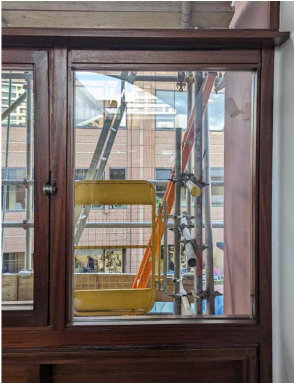
Internal view of trickle vent
